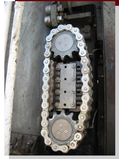
Drive Chain for Elevator Operation
